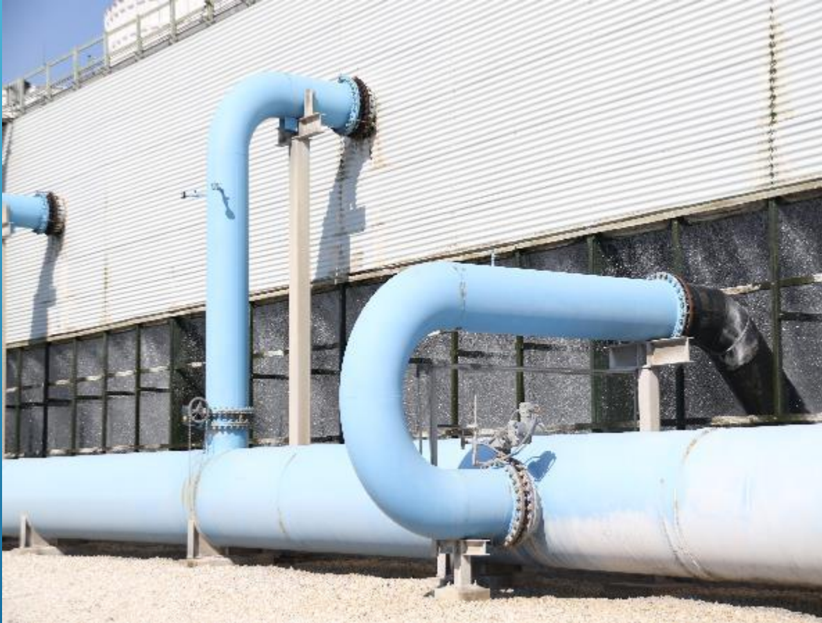
Cooling Tower Bypass
