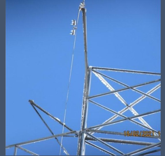
Static Support Damage
